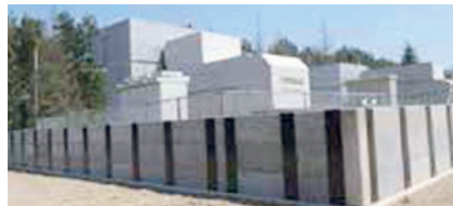
Photo: Water-resistant wall completed for private power generation facility at Senen Purification Plant
