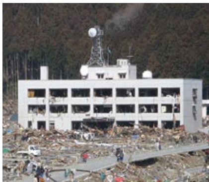
Photo: Damaged prefectural government office building (Minamisanriku Town)
